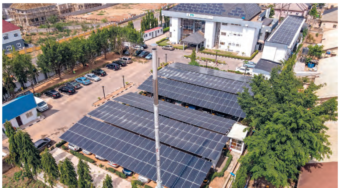
Solar panel systems installed at NRL, Gaduwa
